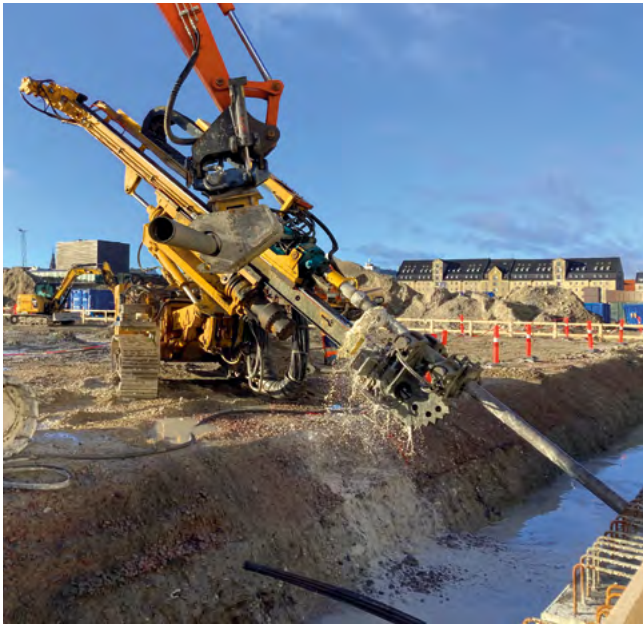
Operaparken, Copenhagen, Denmark Tie-back of a diaphragm wall in two anchor layers with a total of 186 temporary strand anchors.
