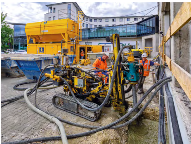
Strengthening the foundation of an industrial building, Munich, Germany As a reinforcement measure, 130 columns were installed up to a depth of approx. 8 m using PI
