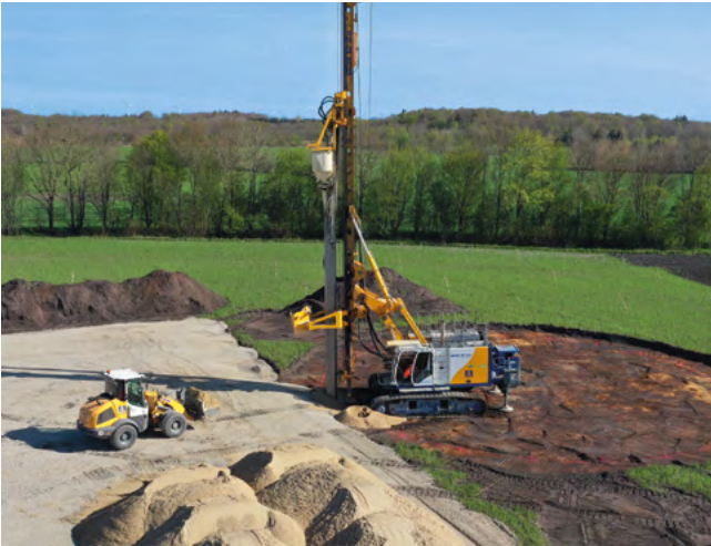
Wind park, Silberstedt, Germany For the foundation of several wind turbines, a total of 3,200 m of vibration replacement were carried out.
