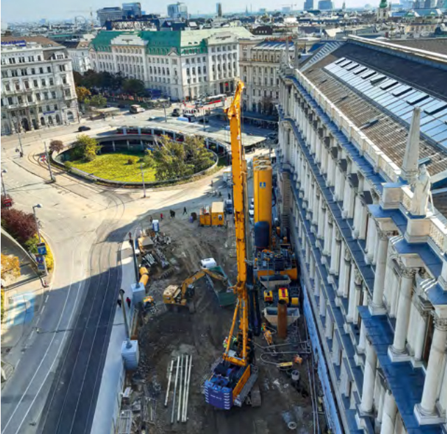
Subway line crossing, Vienna, Austria Construction of roughly 35,000 m of bored piles with varying diameters of up to 1,180 mm and drilling depths of up to 61 m.
