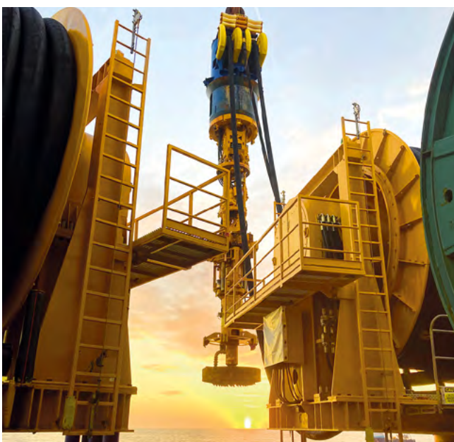
Offshore wind park, Saint-Brieuc, France Using the Dive Drill CU 40, bore holes are constructed up to 47 m deep with a diameter of 3 m.
