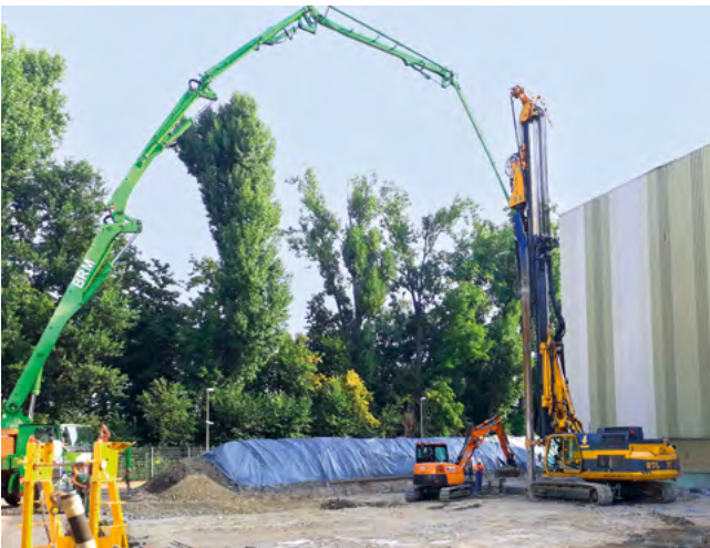
Logistics Center, Karlsruhe, Germany For the foundation work on a logistics center, Bauer carried out 2,700 m of vibro concrete columns.
