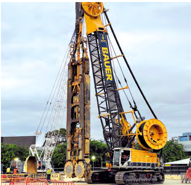
Hobson Bay, Melbourne, Australia Construction of two shafts using an MC 96 duty-cycle crane with a BC 48 trench cutter.
