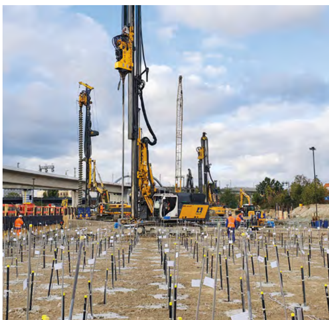
Quartier Heidestraße, Berlin, Germany Execution of 16,000 m 2 of LWS silicate gel base by means of pore injection.
