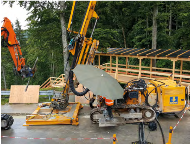
Rosshaupten Dam, Germany Installation of a rock grouting curtain up to a maximum depth of 91 m.
