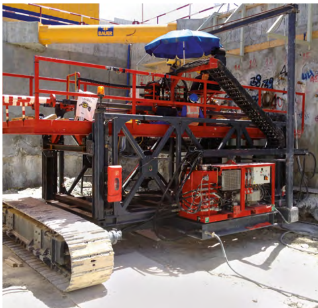
Pedestrian tunnel, Doha, Qatar Controlled drilling for sealing and stabilizing injection in a 90-m pedestrian tunnel.
