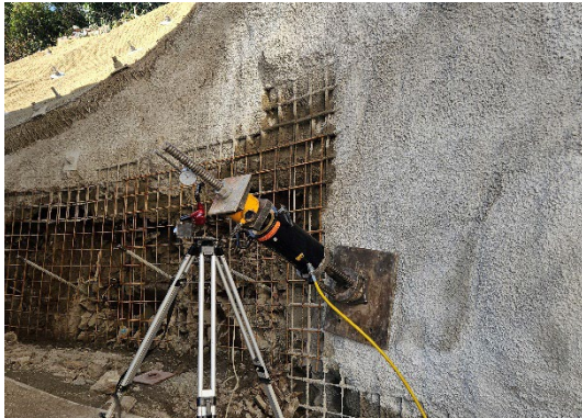
(2) Following the dismantling of the historic masonry, the slope itself is stabilized using a shotcrete shell and anchors.
