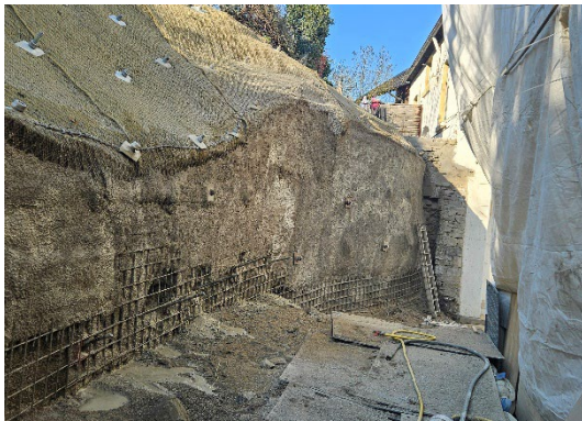
(3) A total of approximately 150 m 2 will be secured with 75 tons of shotcrete.
