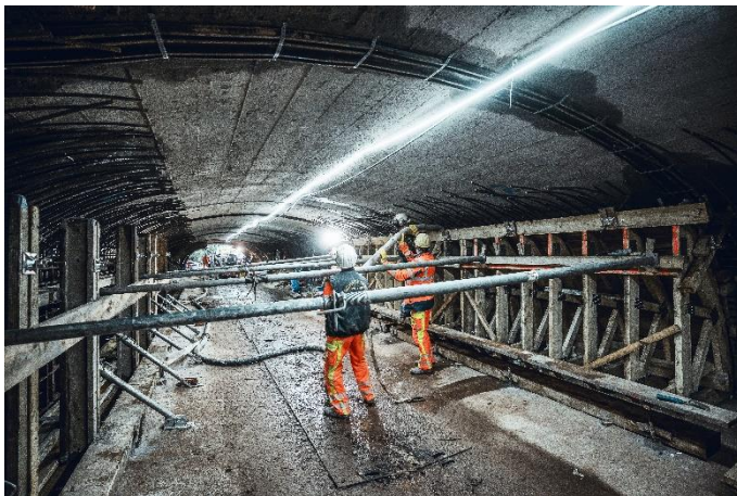
(1) Rehabilitation work on the 160 m long Holzminde tunnel is carried out in tight spaces.
