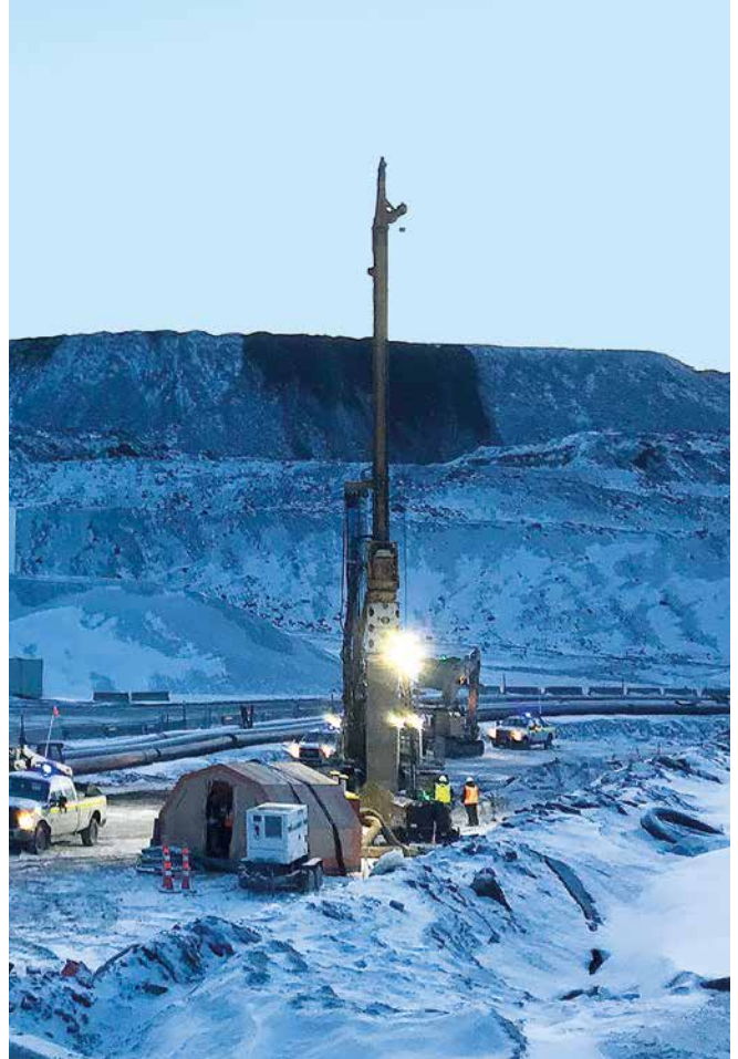
Around 170 km north of the Arctic Circle, Bauer carried out field tests using the jet grouting and cutter soil mixing methods.
