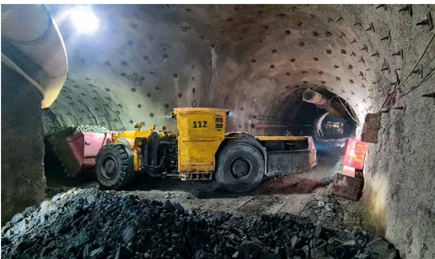
More than 9,000 m of tunneling work has been executed so far in the chrome ore mine in Kazakhstan.
