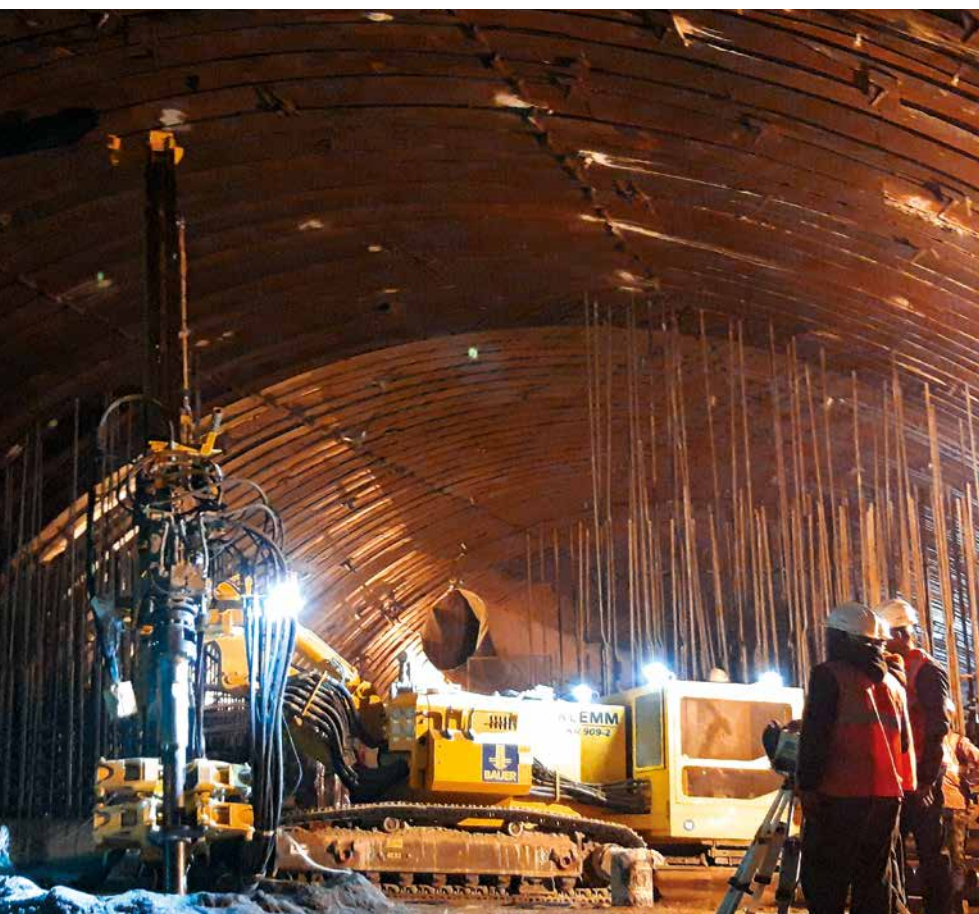
For the hydroelectric power plant Punatsangchhu-II in Bhutan, Bauer executed 19,959 m of drilling with soil and rock grouting for stabilization of the subsoil as well as 18,908 m of ground anchor as tie-back.
