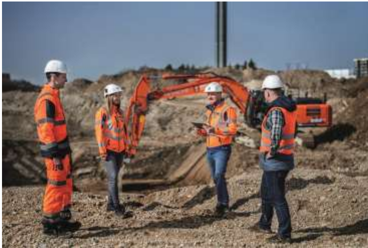
(3) The project team on site: (from left to right) excavator driver Thomas Erwert, site manager Rosa Arystanbaeva, senior foreman Erwin Resch and operations manager Jan Uhlig.
